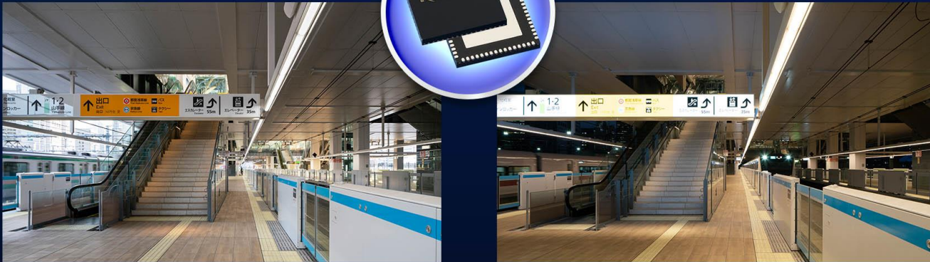
Lighting System at the New Takanawa Gateway Station For Platforms in Tokyo (Left: Daylight Color, Right: Warm White Color)
